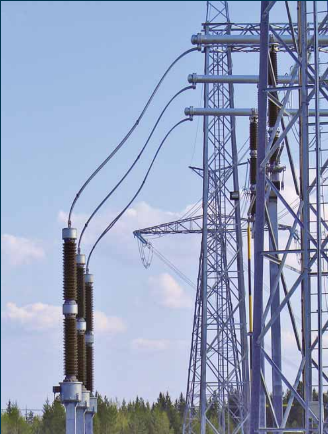
› 420 kV Capacitive voltage transformers. Fingrid, Visulahti (Finland).
